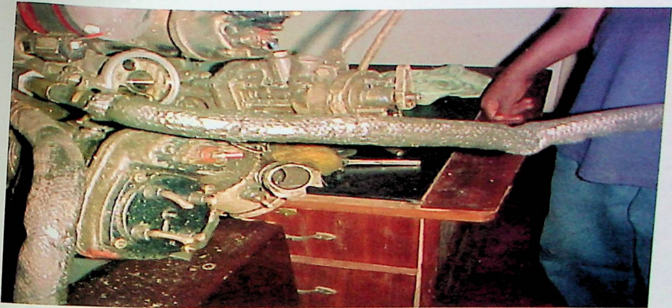
APPDX 5.4A Picture of the canvass conduit, housing the accessory gearbox's broken high pressure hose
